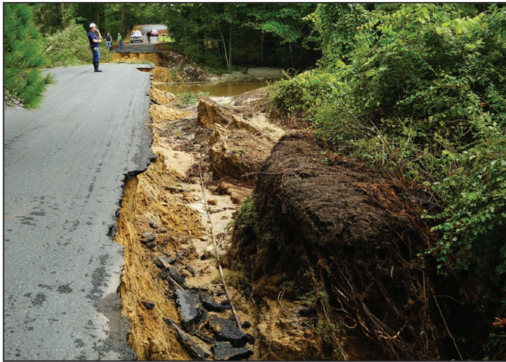
The sides of Hillsborough Drive are washed away after a storm dropped more than 10 inches of rain in less than 24 hours. A utility cable can be seen among the debris.
