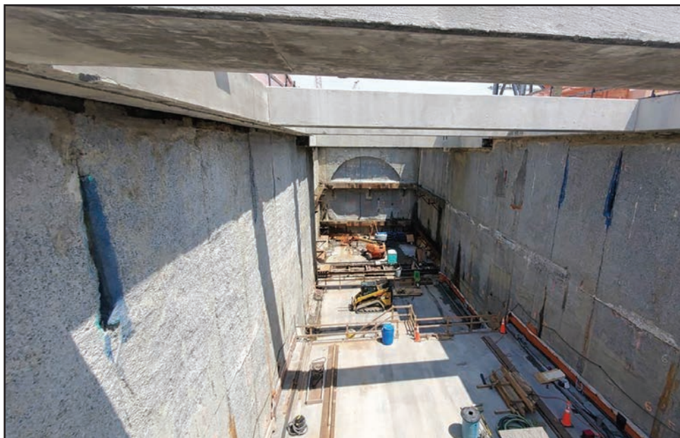
The launch pit for the tunnel boring machine is shown from the inside. The launch pit is approximately 60 feet deep and 50 feet wide. The circle that will align with the cylindrical shape of the tunnel boring machine is 42 feet wide. Photo courtesy of the Chesapeake Bay Bridge-Tunnel.
