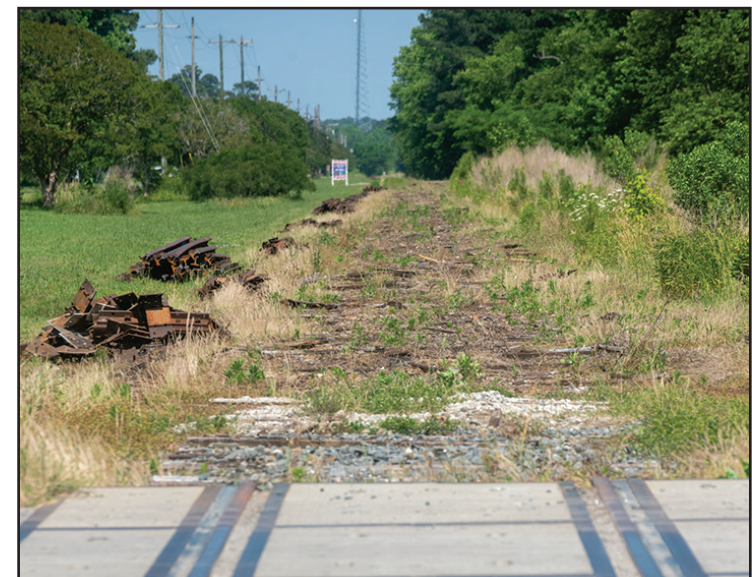
The tracks of a largely unused, high-speed crossing on Cassatt Parkway end at the now empty roadbed where railroad tracks were recently removed. The roadbed will be converted to a bike path from Cape Charles to Route 13, at a cost of over $2 million.
