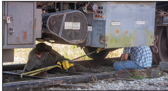
Workers use a come-along under the car to pull a special short section of track into place. The railcar was later rolled forward until one of its trucks rested on the section. Then, the nearby end of the car was lifted, and the truck and section of track pulled out.
