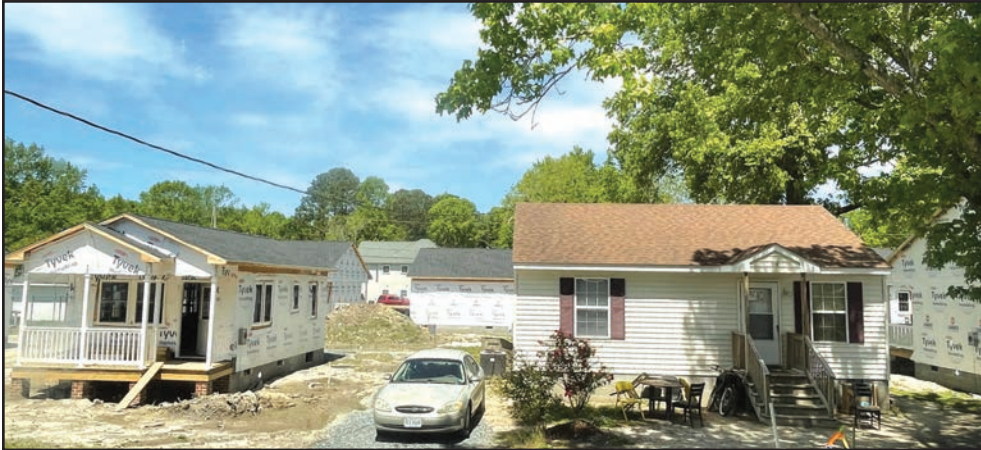
A tiny home is under construction next to an existing two-bedroom home in New Road. Photo by Stefanie Jackson.
