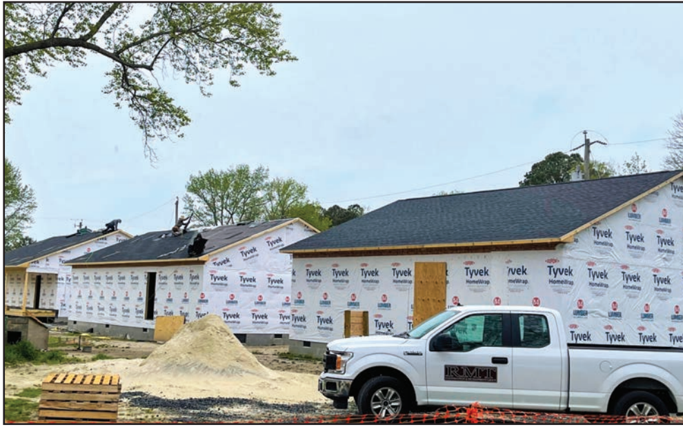
Construction of new houses is in progress in Exmore's New Road community. Photo by Stefanie Jackson.
