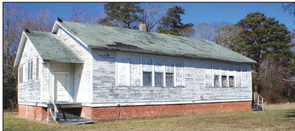
New Boston Elementary School, built in 1923 and opened in 1924, is one of four Rosenwald schools built on the Eastern Shore.
