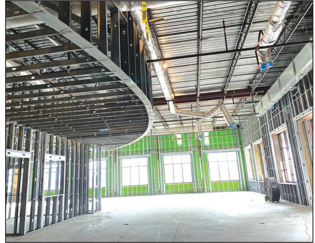
An interior view of the Eastern Shore of Virginia Regional Library and Heritage Center construction site, taken Feb. 23. Photo courtesy of Eastern Shore Public Library.
