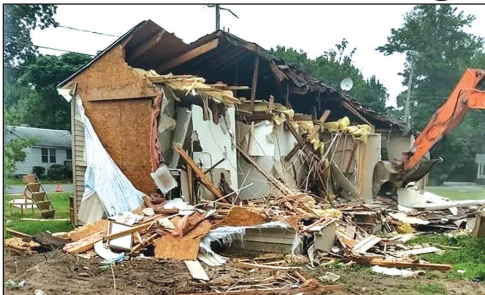
A house in the New Road community in Exmore is demolished to make way for one of six new homes that will be either 3D-printed or stick-built. Photo courtesy of Ava Wise.
