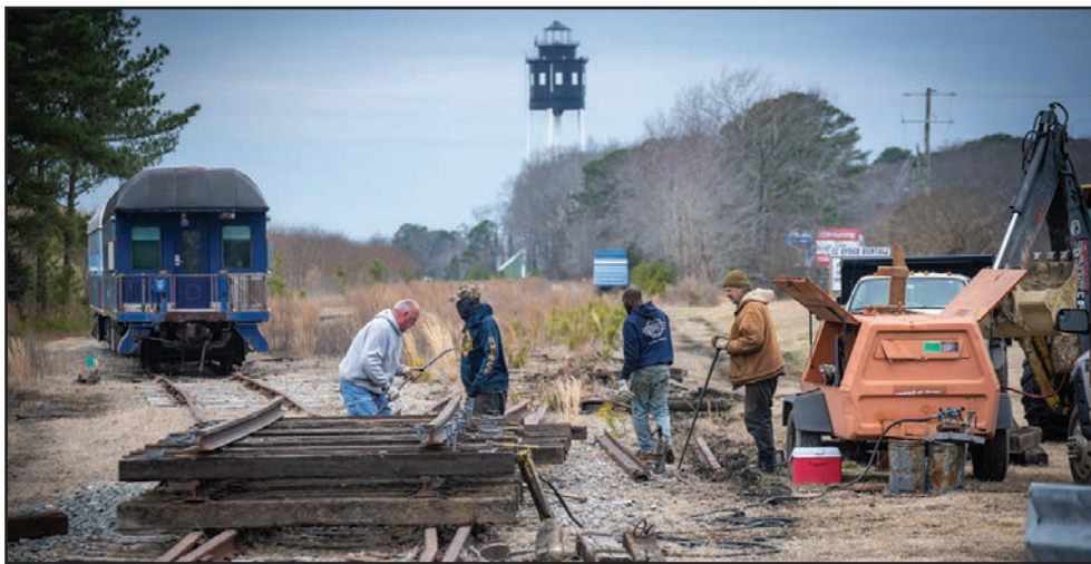
New portable, track panels lie under construction alongside Stone Road outside Cape Charles. The panel will support the cars at left when they are moved.
