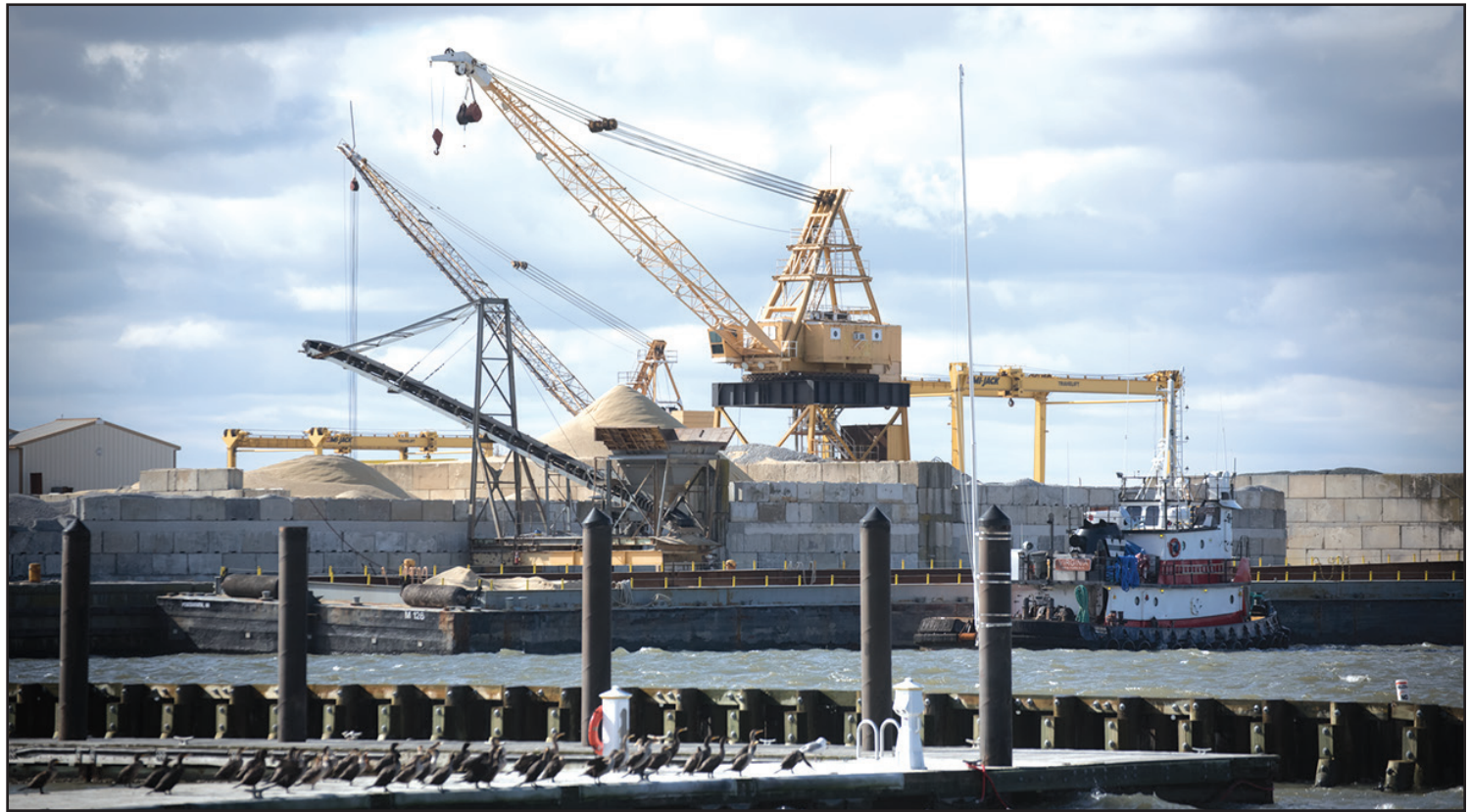
Cranes and docks of Coastal Precast Systems rise beyond slips for recreational boaters in Cape Charles Town Harbor.
