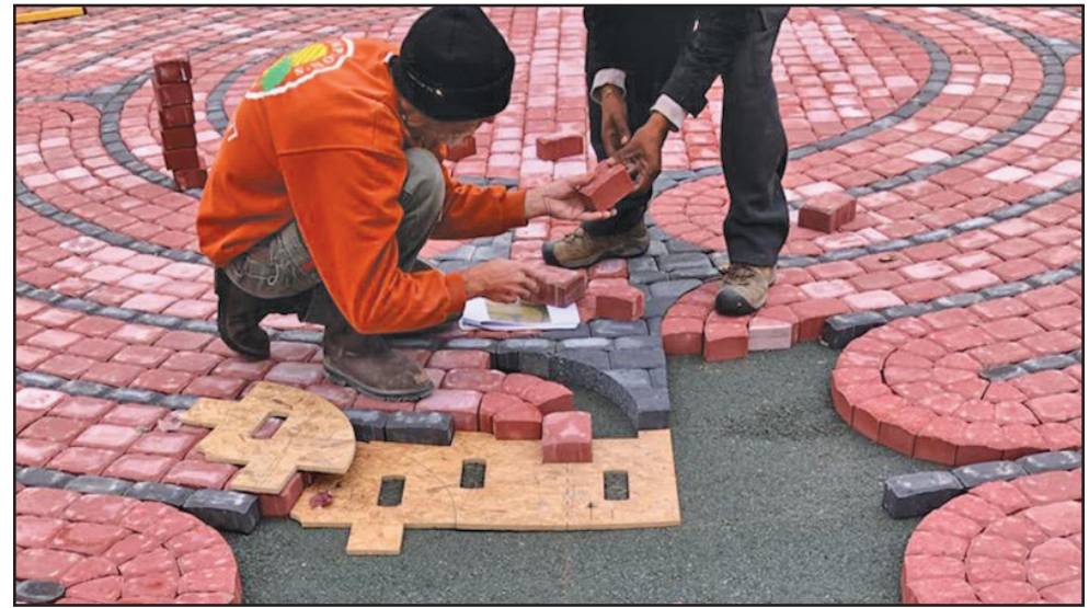
Construction of the labyrinth at McMath Park. Photo courtesy of Billye D. Custis.
