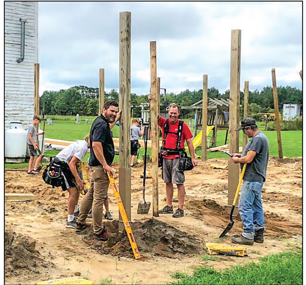
Pungoteague Community Church and Men on Mission volunteers pause during the early stages of framing the new storage building Friday, Sept. 11. From left are Frank Pennell, Darren Lane, and Pastor Bobby Huether. Submitted photo.
