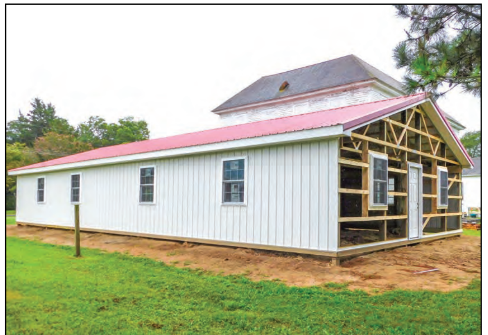
With the help of Men on Mission, construction is nearly complete. Two exterior walls and a concrete floor are needed. Photo by Stefanie Jackson.
