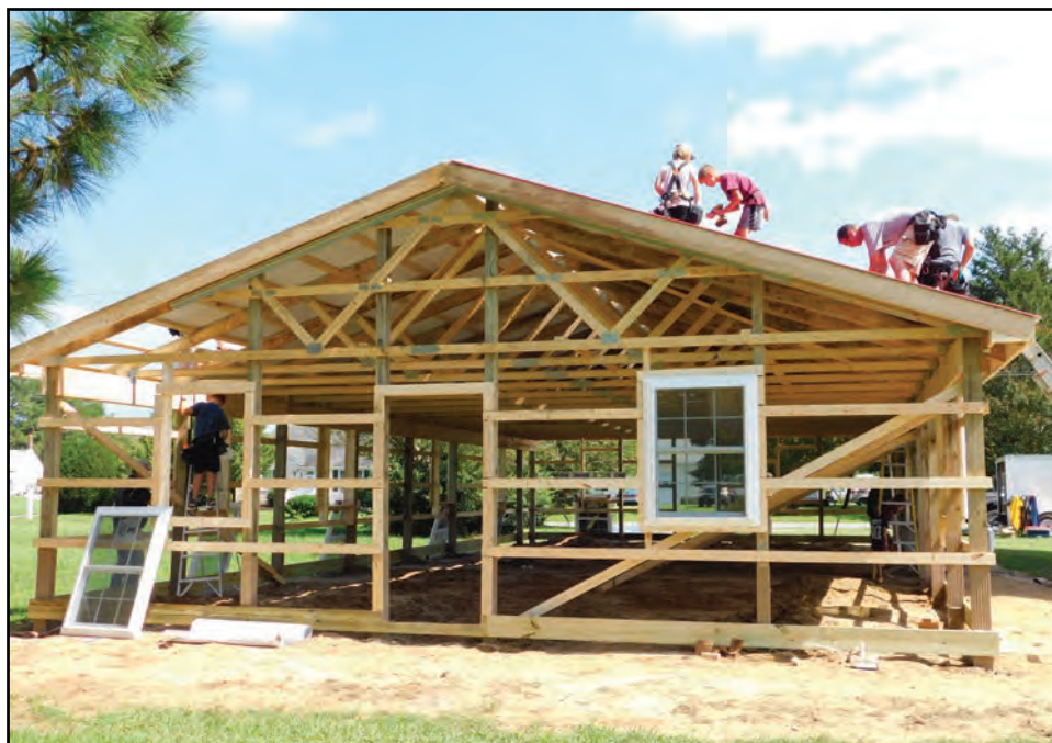
The group may be called Men on Mission, but the kids volunteer their time and skills, too. With the frame complete, work on roofing and window installation begins. Photo by Stefanie Jackson.
