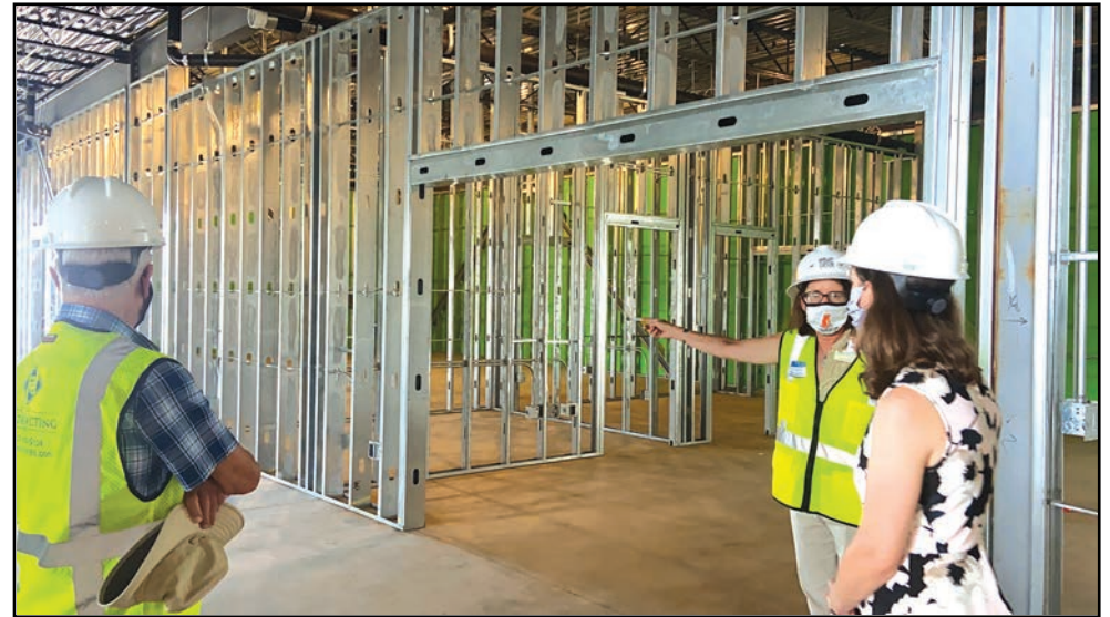
Cara Burton, Eastern Shore Public Library director, gestures as she leads Rep. Elaine Luria and others on a tour of the new library under construction in Parksley on Thursday, Sept. 3. The area that will be the Eastern Shore of Virginia Heritage Center is behind Burton. Photo by Carol Vaughn.
