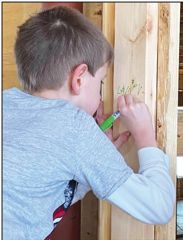
Levi, the grandson of Eastern Shore Yacht & Country Club members John and Kate Morgan, signs a stud of the new clubhouse now under construction. Members held a reception Saturday to pen messages on the studs. Photo by Bill Sterling.
