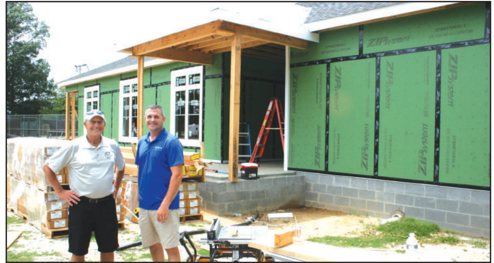
Eastern Shore Yacht and Country Club board member Eric Dodge, left, and Jamie Hammond of Gateway Builders in Pocomoke City, Md., are pictured in front of the new sports facility under construction at the club, expected to be in use by Labor Day weekend.
