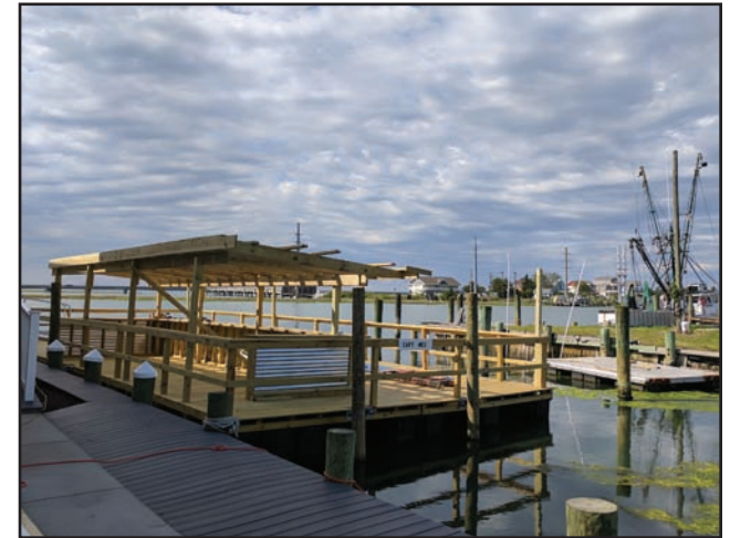
The Ropewalk Chincoteague’s barge bar is still under construction and set to open later this summer. It is billed as Chincoteague’s only floating barge bar.
