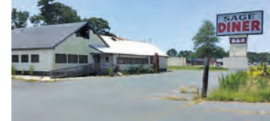
8,200 sf. fire-damaged former restaurant on 2.5 acres.
