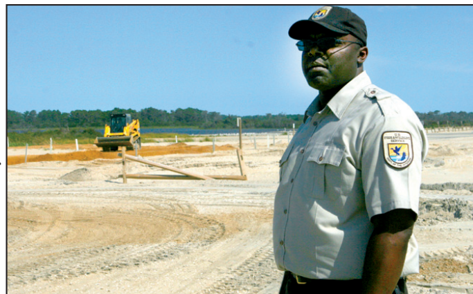
Michael Dixon, visitor services manager for Chincoteague National Wildlife Refuge, surveys beach damage from Hurricane Irene while a loader spreads clay on the entrance circle.
