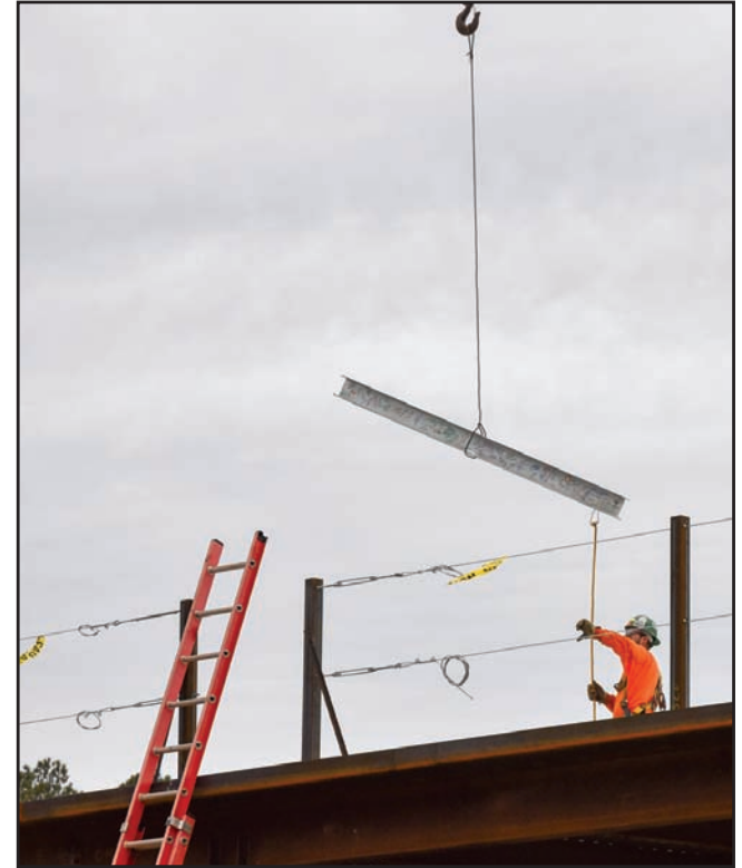
The final beam, with signatures, is put into place atop the Riverside Shore Cancer Center.
