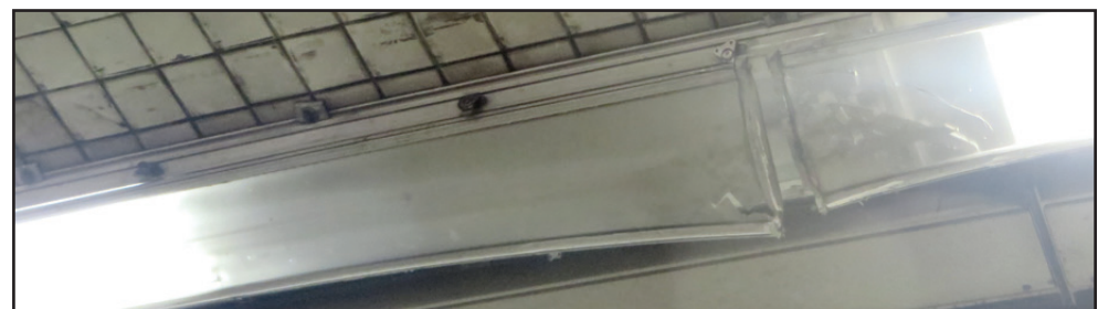
Pictured is some of the damage done in CBBT tunnel by truck
